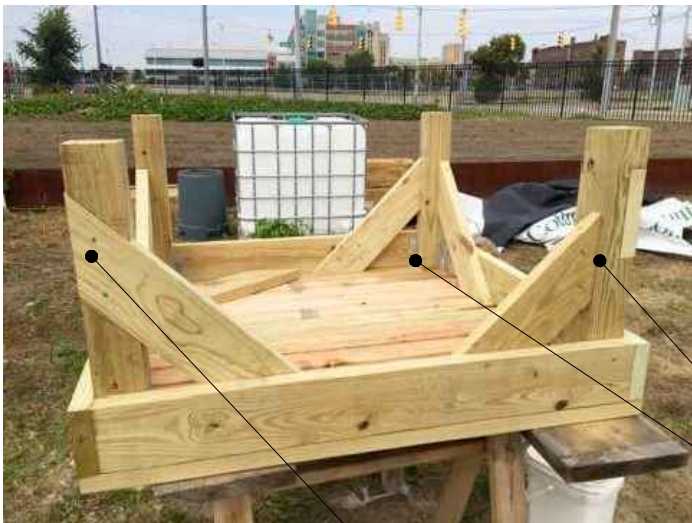
#4 Notch one face of each post to receive cross brace as shown
